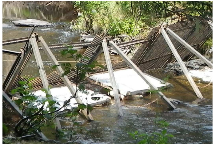
Figure 20. Drop-down panels installed in the weir. Note the shorter pipes at the bottom of the large opening.
