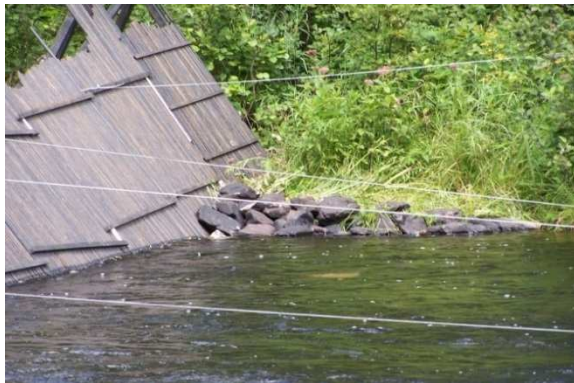
Figure 19. Rip-rap material piled along the streambank to reduce potential erosion during high flow events.
